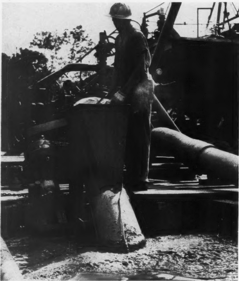
DUMPING DRY mud materials into the new mud mixer is fast and easy; steam turbine-driven propellers in the mixer and on the bottom of the pit keep the mud constantly agitated.
